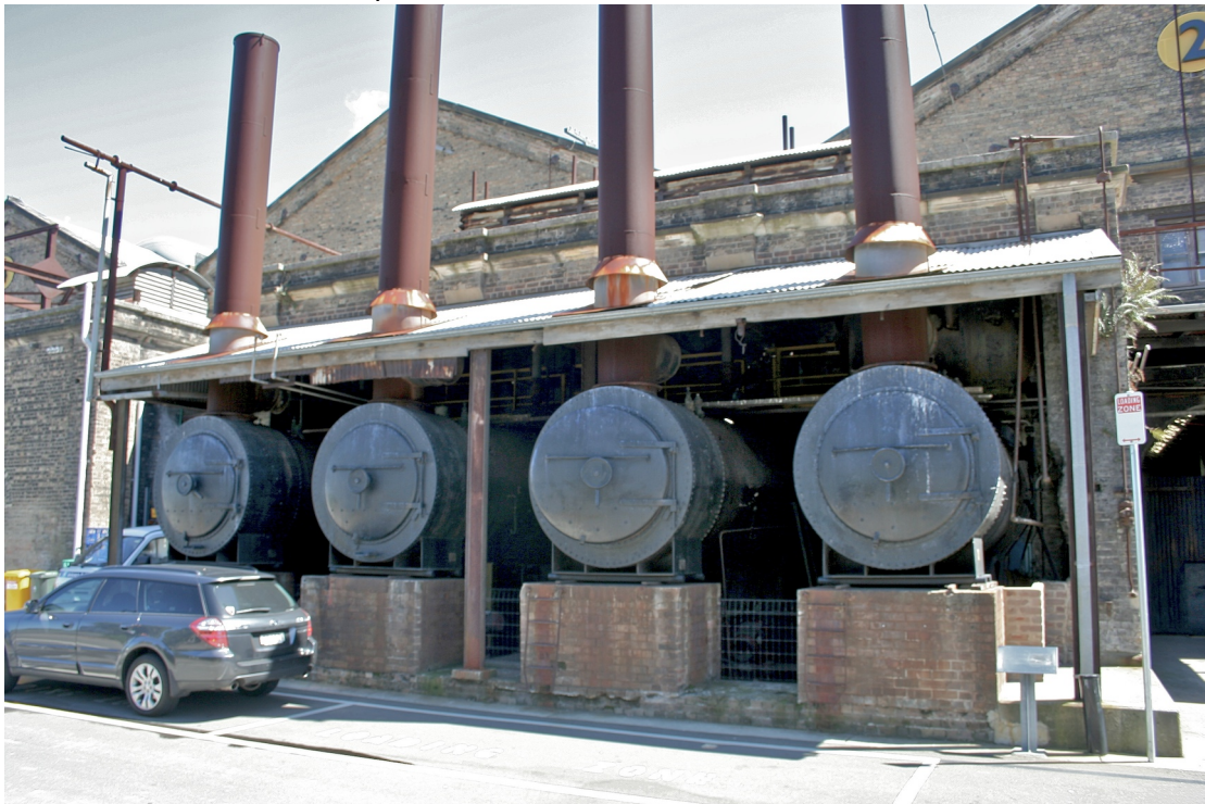
Figure 11 - The boilers located in the Bay 2 Annex
